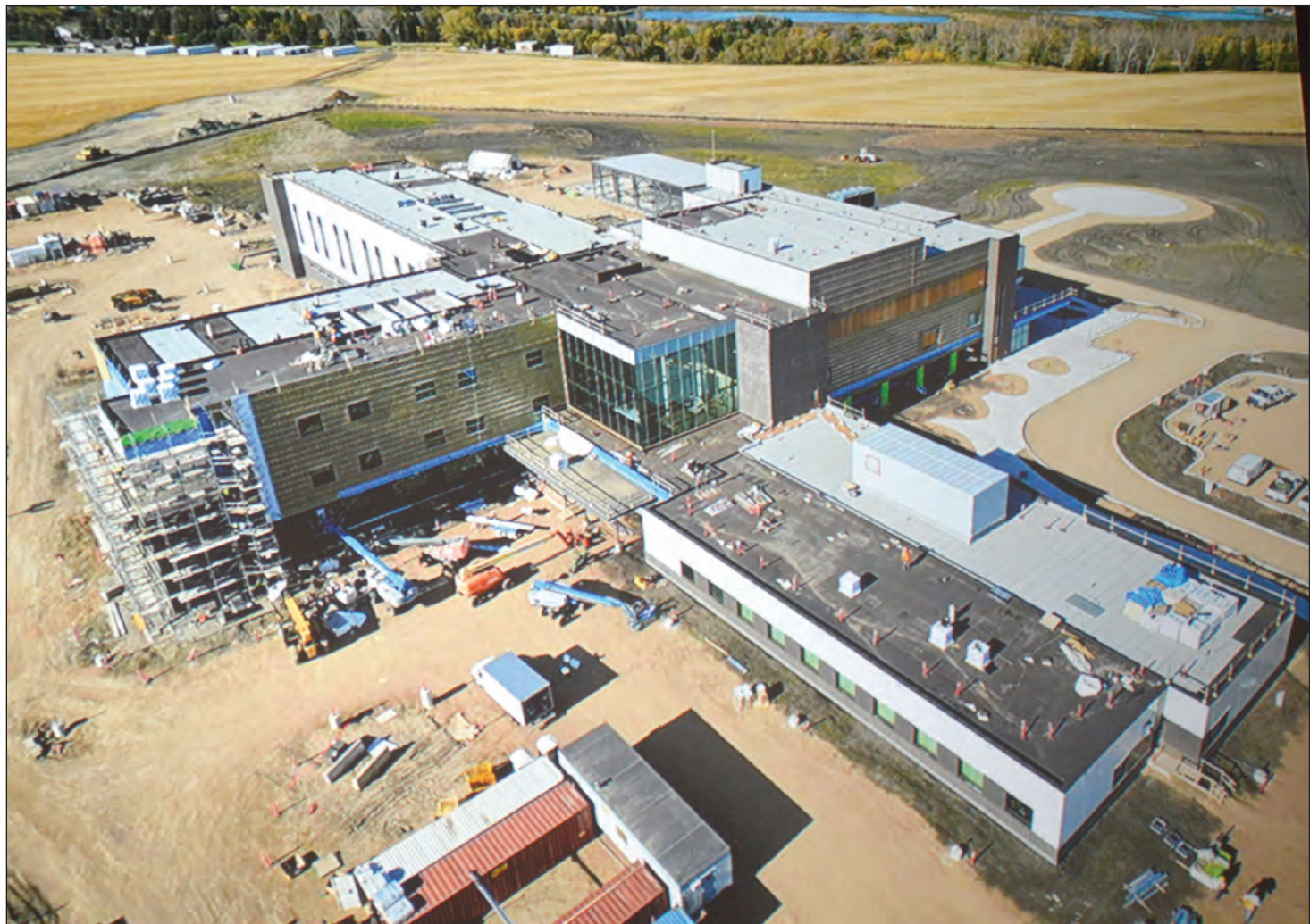
PRAIRIE MOUNTAIN HEALTH AND LM ARCHITECTURAL PRESENTATION Prairie Mountain Health and LM Architectural provided an update on the construction of the new Neepawa Health Centre (hospital) on Oct. 24.
